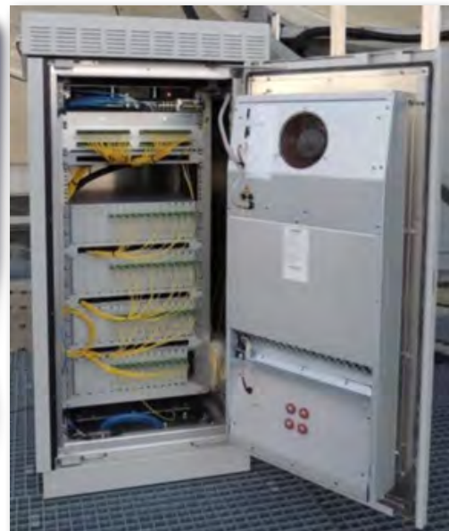
Rack Shelter with devices for electro-optical conversion (Source: DEV Systemtechnik)
